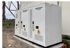
99.12kWp PV 120kW/416kWh Liangmaoshan
